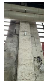
Figure 4. One of six installed UWB indoor Anchors in the test area
