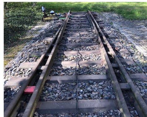
Figure 20. Real-world test investigations into the use of leaky waveguide cables for localization and information transmission in the rail sector
