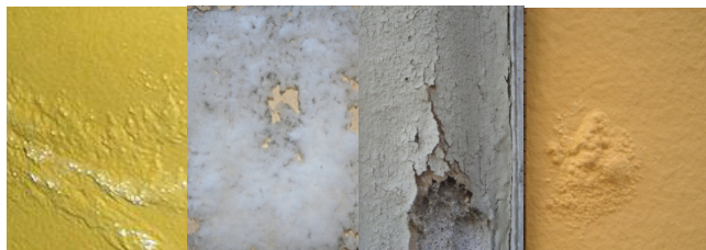
Figure 1. Swelling, efflorescence, cracking and blistering [17].
