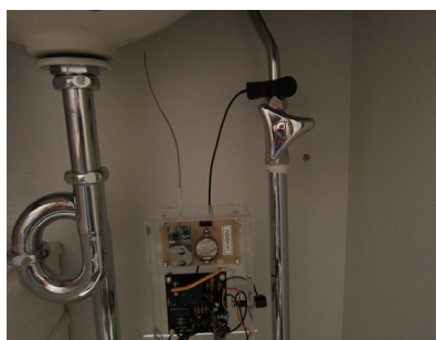
Figure 3. The water flow sensor is installed at the sink. The vibration microphone is clipped to a water pipe near the faucet.
