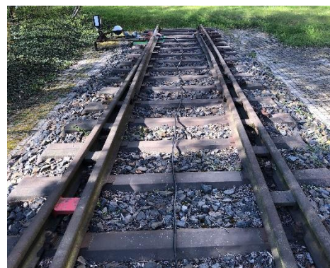
Figure 20. Real-world test investigations into the use of leaky waveguide cables for localization and information transmission in the rail sector
