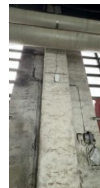
Figure 4. One of six installed UWB indoor Anchors in the test area
