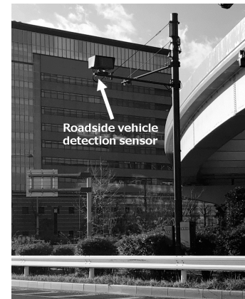
Figure 1. Roadside vehicle detection sensor.
