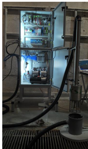
Figure 2. Measuring system for the monitoring of process water, consisting of control box (a), Measuring lance (b) and measuring barrel (c)
